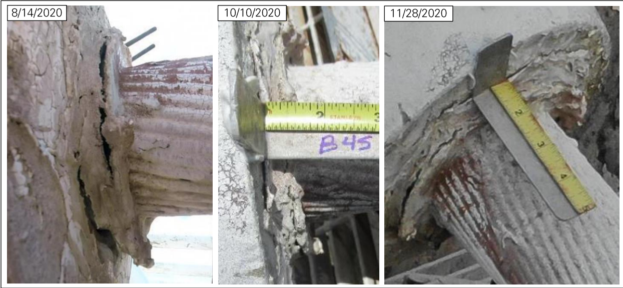
Figure 33: Cable slip at socket B4S_T (left and right photos: NAIC Arecibo Observatory, a facility of the NSF; center photo: WJE 13 ).
