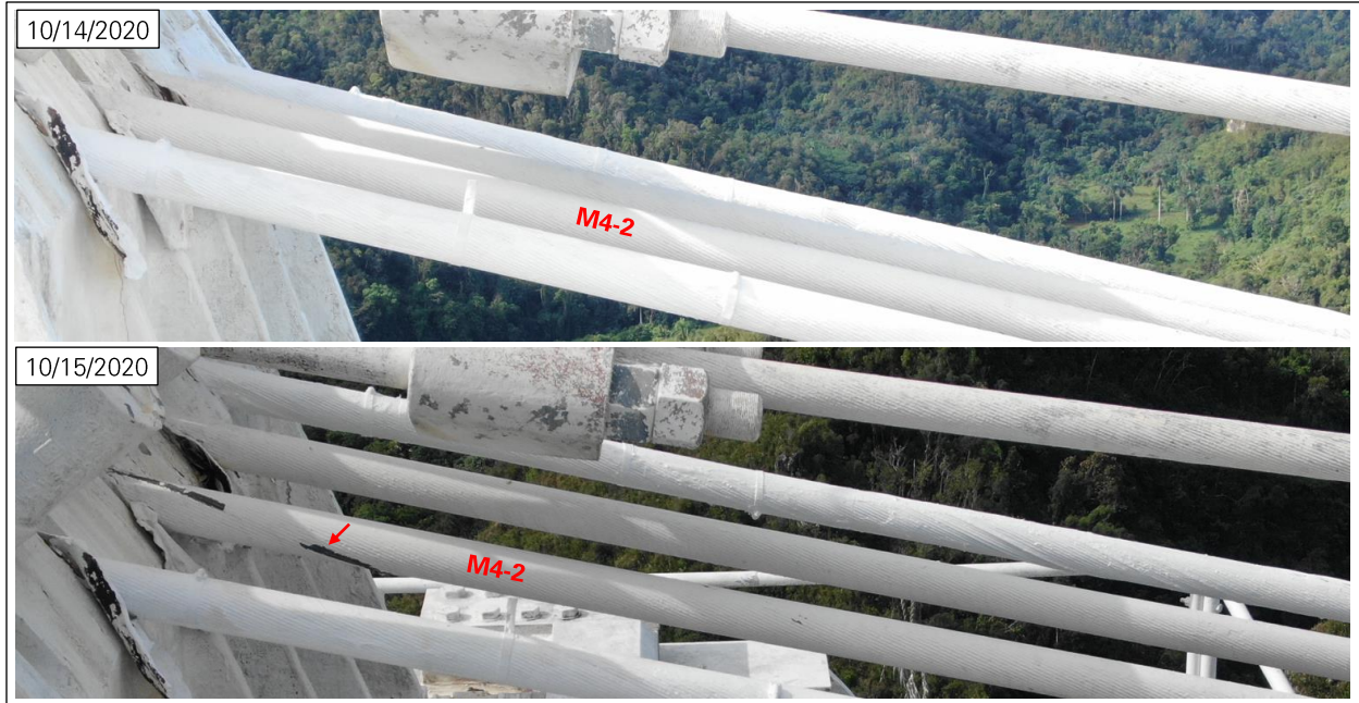
Figure 10: New wire break in M4-2 on October 15, 2020 (photos: NAIC Arecibo Observatory, a facility of the NSF).
