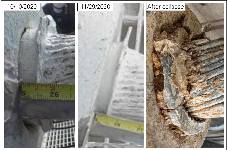
Figure 26: Cable slip at socket M12W_T (left photo: WJE 12 ; center photo: NAIC Arcibo Observatory, a facility of the NSF).
