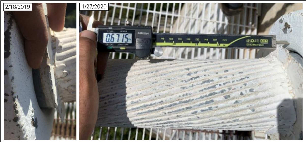
Figure 23: Cable slip at socket M12E_T (photos: NAIC Arecibo Observatory, a facility of the NSF).
