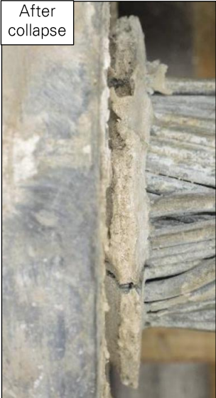
Figure 29: Cable slip at socket M8S_P.
