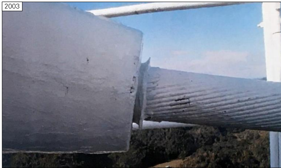
Figure 19: Cable slip at socket M4S_T (photo: Ammann & Whitney 8 ).
