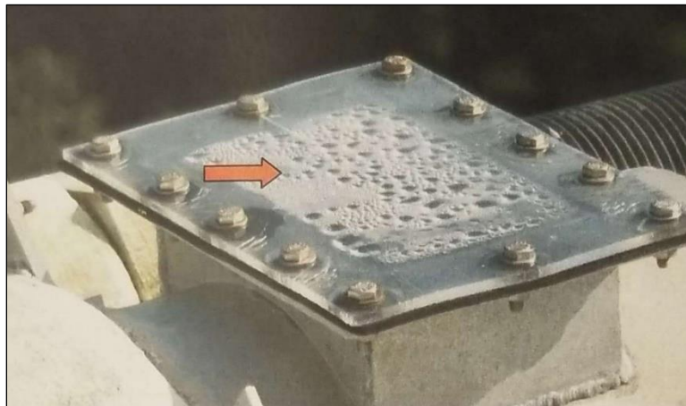
Figure 8: Condensation inside dry air sleeve on cable M4N in 2011 (photos: Amman & Whitney 5 ).
