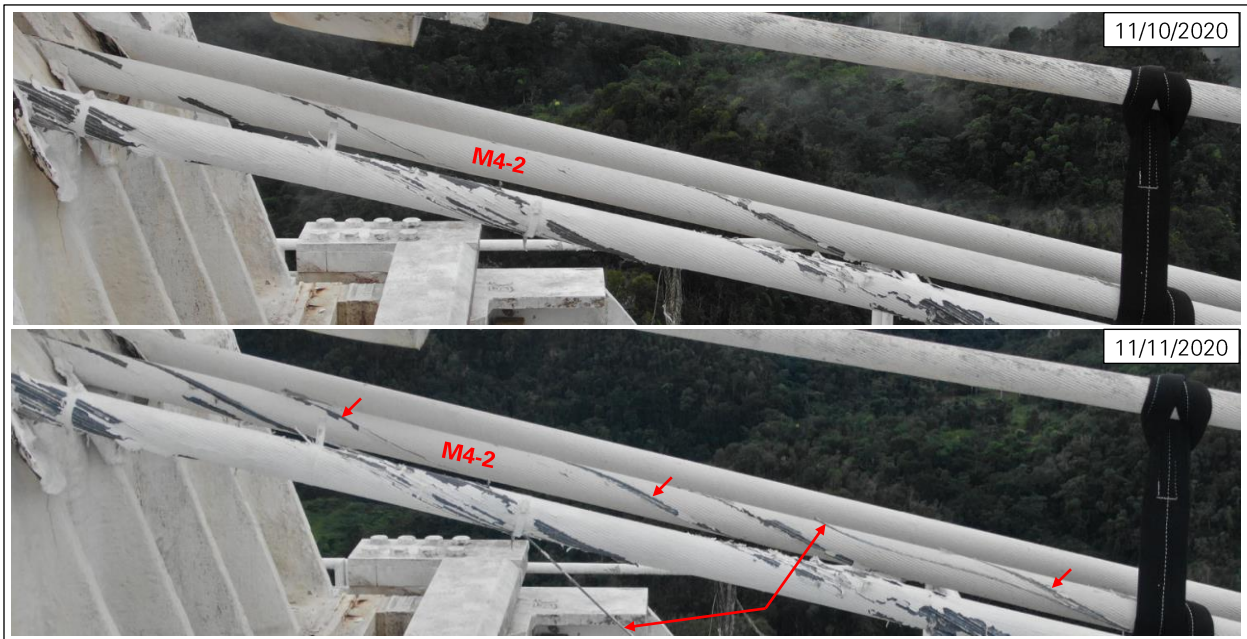
Figure 21: New wire break in M4-2 on November 11, 2020. The break occurred away from the socket. (Photos: NAIC Arecibo Observatory, a facility of the NSF.)
