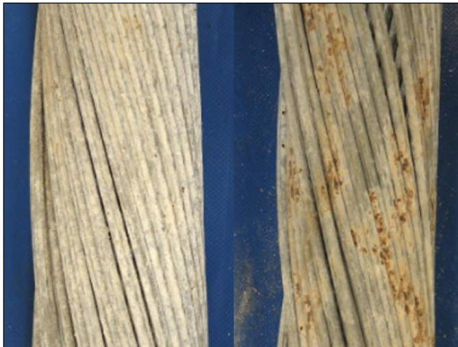
Figure 30: Oxidation of galvanizing zinc (left) and wire steel (right) in second wire layer of an original M4 cable (photos: Socotec).
