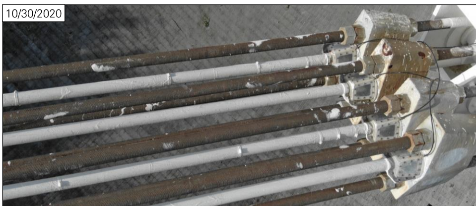
Figure 13: M4 cables near platform on October 30, 2020. No wire is broken. (Photo: NAIC Arecibo Observatory, a facility of the NSF.)
