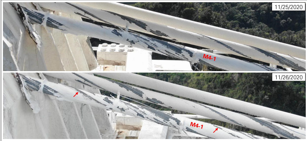
Figure 25: New wire break in M4-1 on November 26, 2020 (photos: NAIC Arecibo Observatory, a facility of the NSF).
