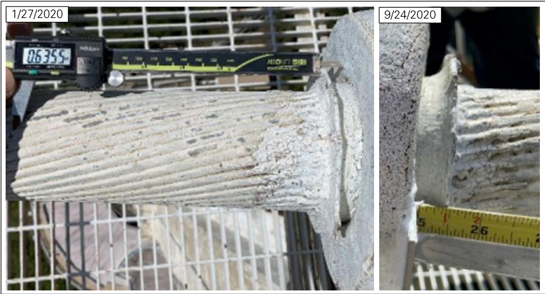
Figure 25: Cable slip at socket M12W_T (left photo: NAIC Arcibo Observatory, a facility of the NSF; right photo: WJE 12 ).
