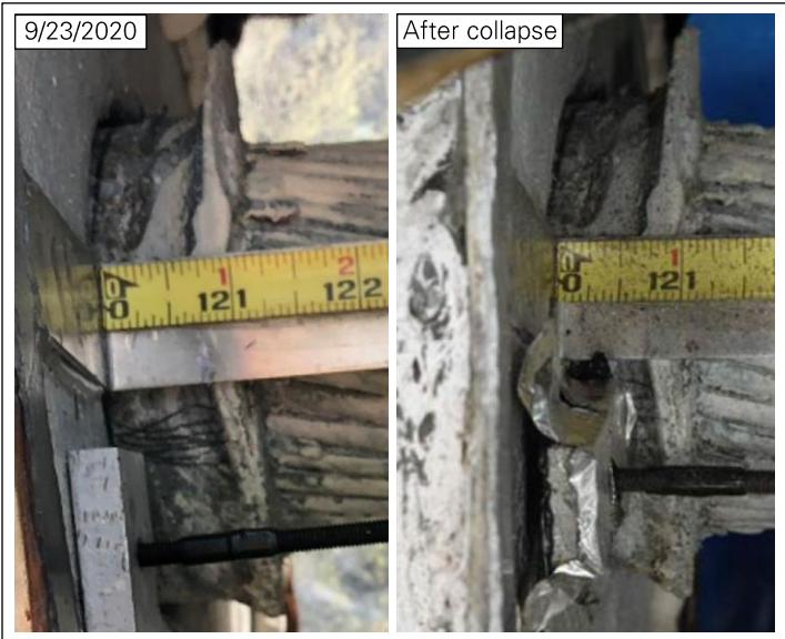
Figure 38: Cable slip at socket B4N_G (left photo: WJE 15 ).
