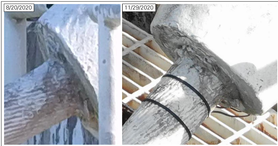
Figure 35: Cable slip at socket B8S_T (photos: NAIC Arecibo Observatory, a facility of the NSF).
