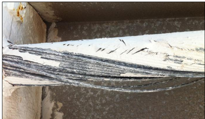
Figure 21: Multiple wire breaks observed at splice near tower end of cable M8-4 on 1/14/2014 (photo: NAIC Arecibo Observatory, a facility of the NSF).
