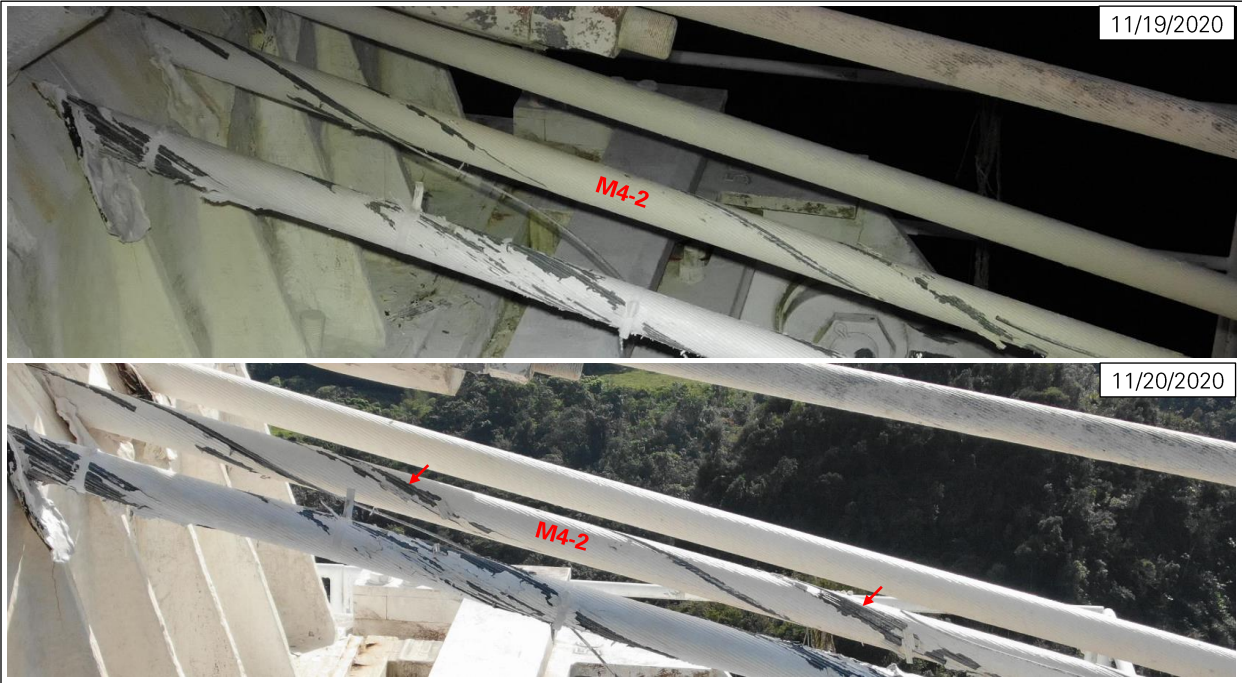
Figure 23: New wire break in M4-2 on November 20, 2020 (photos: NAIC Arecibo Observatory, a facility of the NSF).
