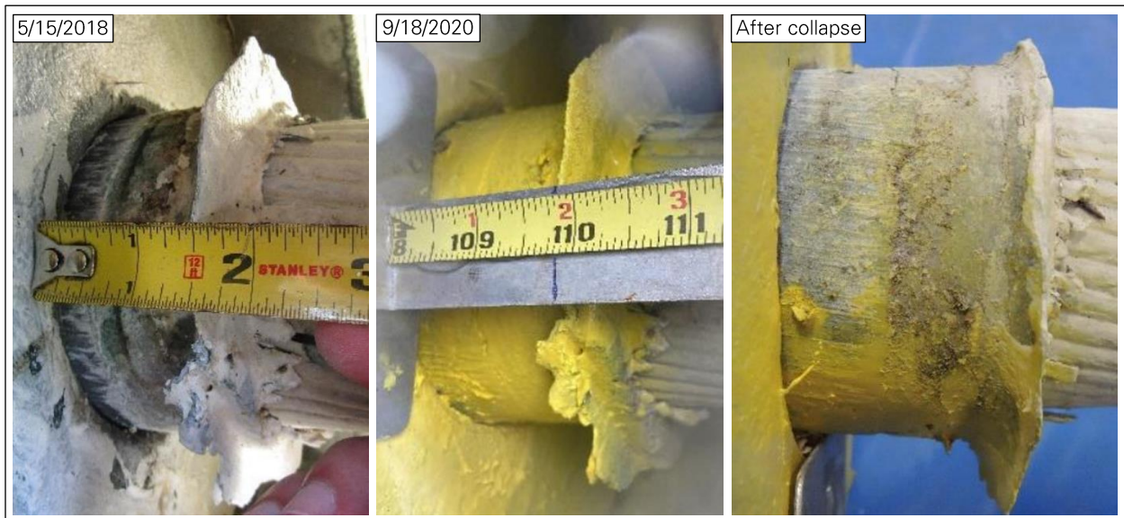
Figure 43: Cable at socket B12W_G (left and center photos: NAIC Arecibo Observatory, a facility of the NSF).
