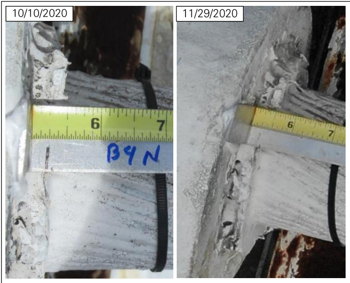
Figure 32: Cable slip at socket B4N_T (left photo: WJE 13 ; right photo: NAIC Arecibo Observatory, a facility of the NSF).
