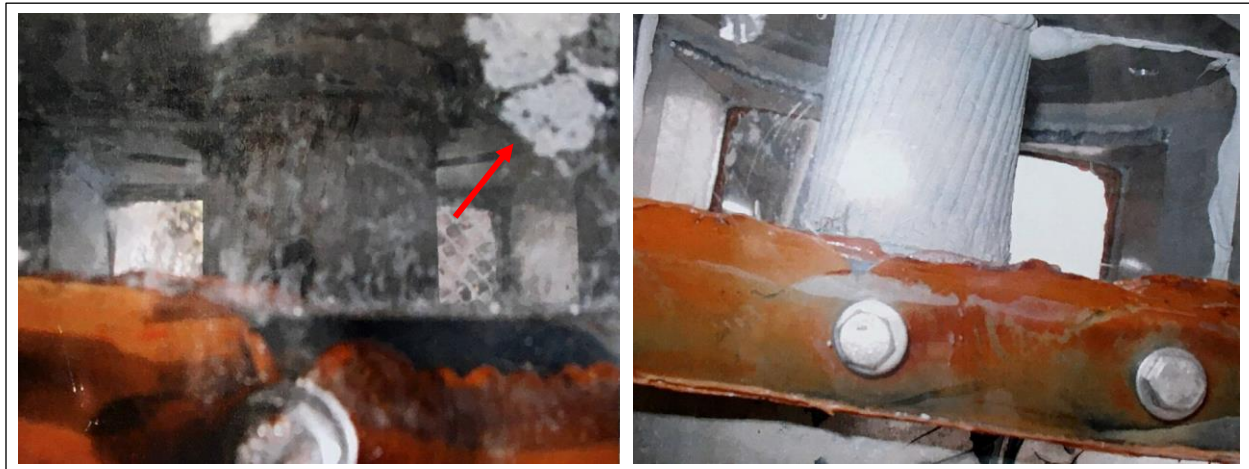
Figure 7: Condensation inside dry air sleeve of cable B4S (left) compared to typical condition of dry air sleeves (right) in 2003 (photos: Amman & Whitney 4 ).
