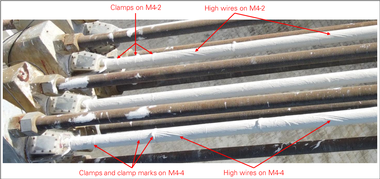
Figure 12: Evidence of past wire breaks at platform end of M4 cables (photo: NAIC Arecibo Observatory, a facility of the NSF).
