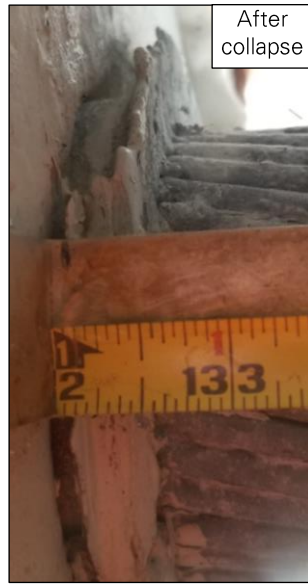
Figure 40: Cable slip at socket B8N_G.
