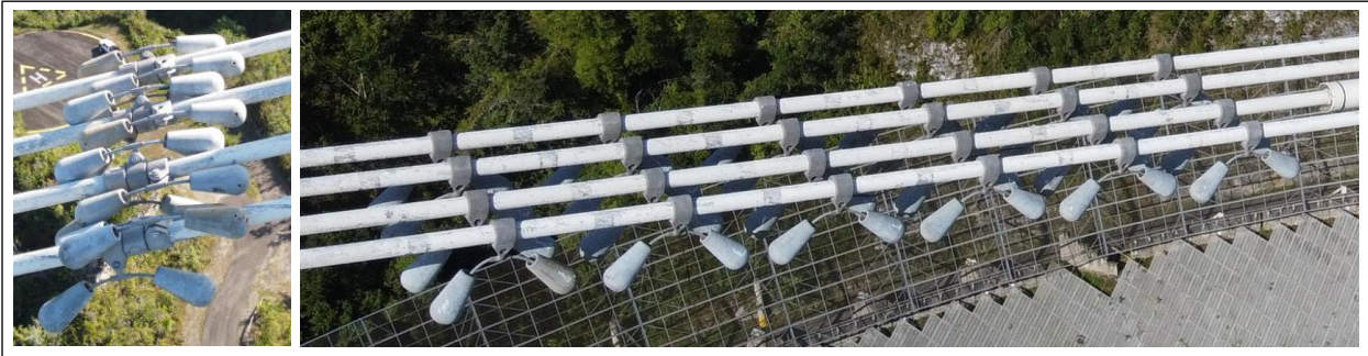
Figure 44: Stockbridge dampers near top (left) and bottom (right) of original M4 cables in 2020 (photos: NAIC Arecibo Observatory, a facility of the NSF).
