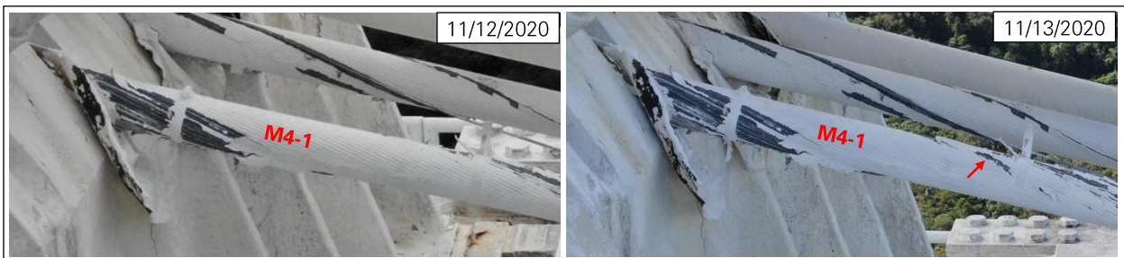
Figure 22: New wire break in M4-1 on November 13, 2020 (photos: NAIC Arecibo Observatory, a facility of the NSF).
