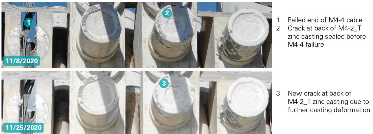
Figure 28: Evidence of socket casting core displacement after second cable failure (photos: NAIC Arecibo Observatory, a facility of the NSF).
