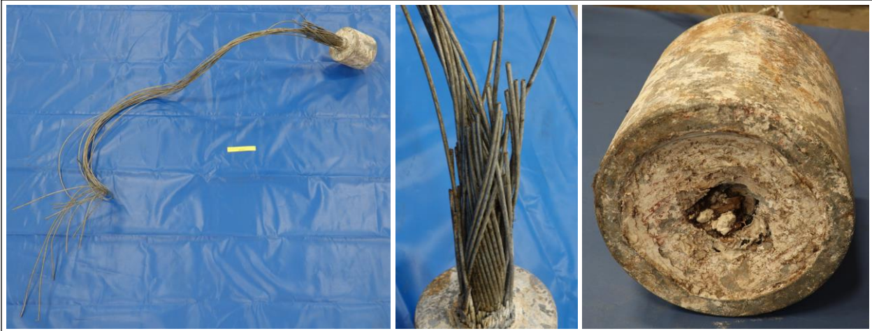
Figure 4: Socket M4-4_T (photos: Socotec).
