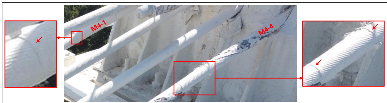
Figure 3: Clamps on M4-1 and M4-2 near Tower 4, likely installed after previous wire breaks. The paint damage on M4-4 corresponds to fresh wire breaks following the M4N failure. (Photo: NAIC Arecibo Observatory, a facility of the NSF.)
