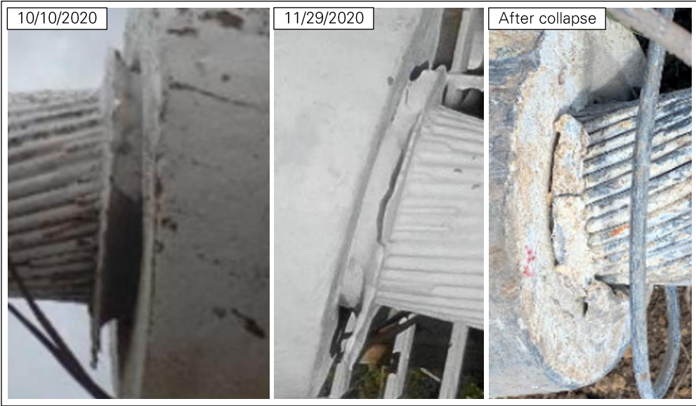
Figure 22: Cable slip at socket M8S_T (left photo: WJE 10 ; center photo: NAIC Arecibo Observatory, a facility of the NSF).
