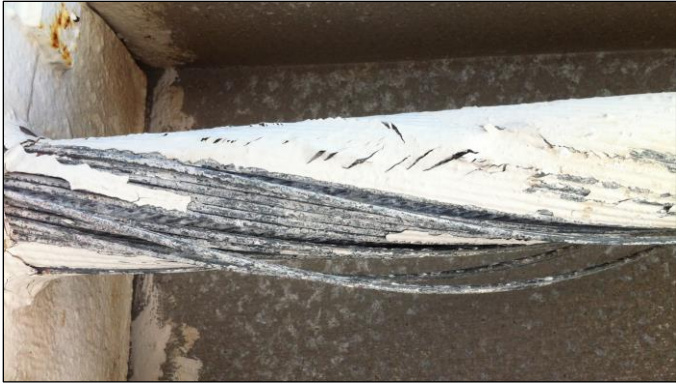
Figure 11: Multiple wire breaks near M8-4 splice discovered on January 14, 2014 (photo: NAIC Arecibo Observatory, a facility of the NSF).
