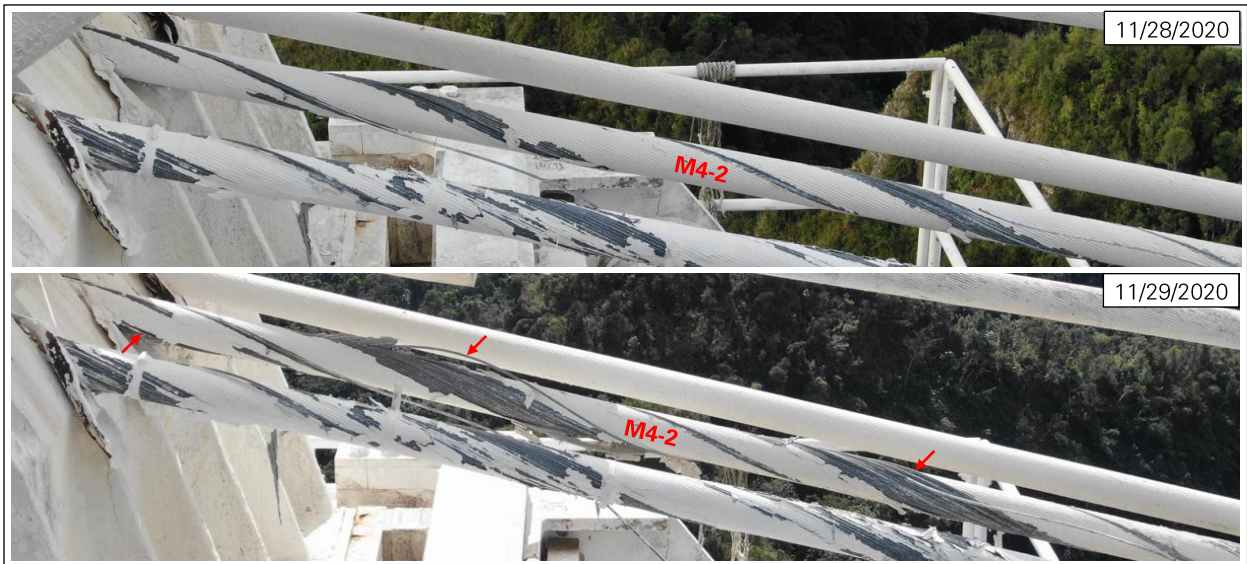
Figure 26: New wire break in M4-2 on November 29, 2020 (photos: NAIC Arecibo Observatory, a facility of the NSF).
