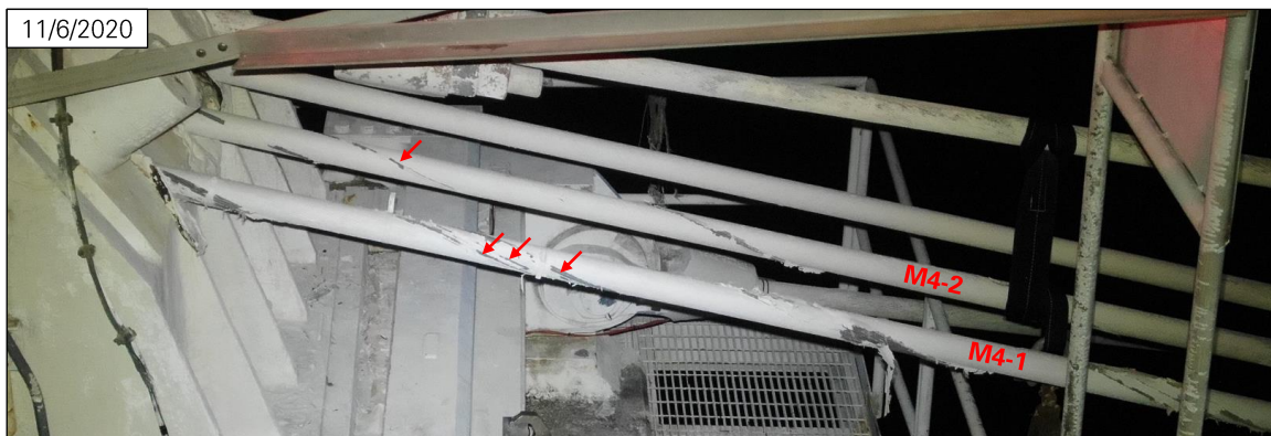
Figure 16: M4 cables near Tower 4 on November 6, 2020, with three new wire breaks in M4-1 and a new wire break in M4-2 (photos: NAIC Arecibo Observatory, a facility of the NSF).
