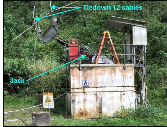
Figure 7: Base of tiedown 12, after telescope collapse.
