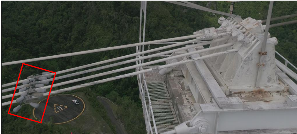
Figure 7: Stockbridge dampers on Tower 4 original mains.
