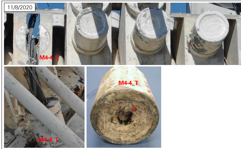
Figure 18: M4 sockets at Tower 4 on November 8, 2020, and socket M4-4_T as recovered after collapse (top and bottom left photos: NAIC Arecibo Observatory, a facility of the NSF; bottom center photo: Socotec).
