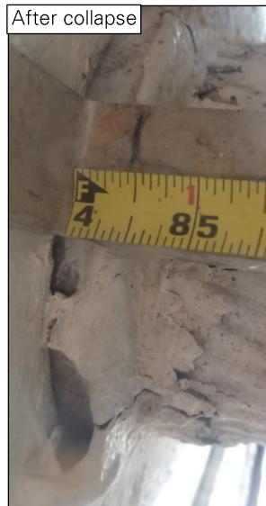
Figure 41: Cable slip at socket B8S_G.
