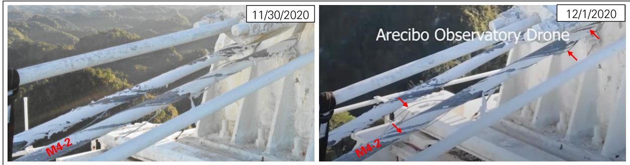
Figure 27: Two new wire breaks in M4-2 on December 1, 2020 (photos: NAIC Arecibo Observatory, a facility of the NSF).
