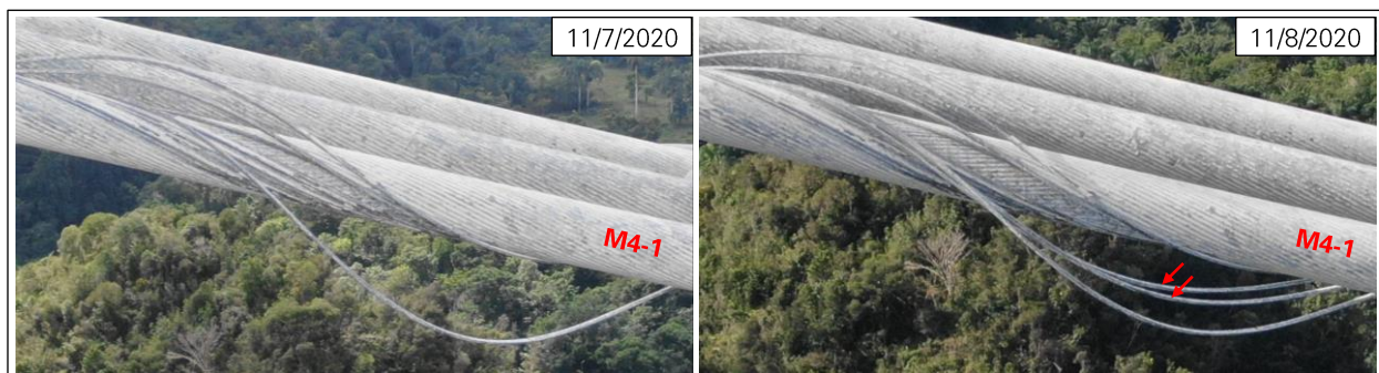
Figure 19: Two new wire breaks in M4-1 on November 8, 2020 (photos: NAIC Arecibo Observatory, a facility of the NSF).
