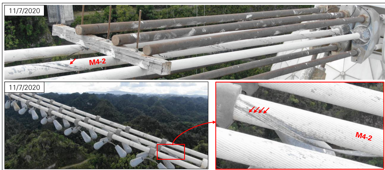
Figure 17: M4 cables near platform on November 7, 2020. Four adjacent wires are broken in M4-2. (Photos: NAIC Arecibo Observatory, a facility of the NSF.)
