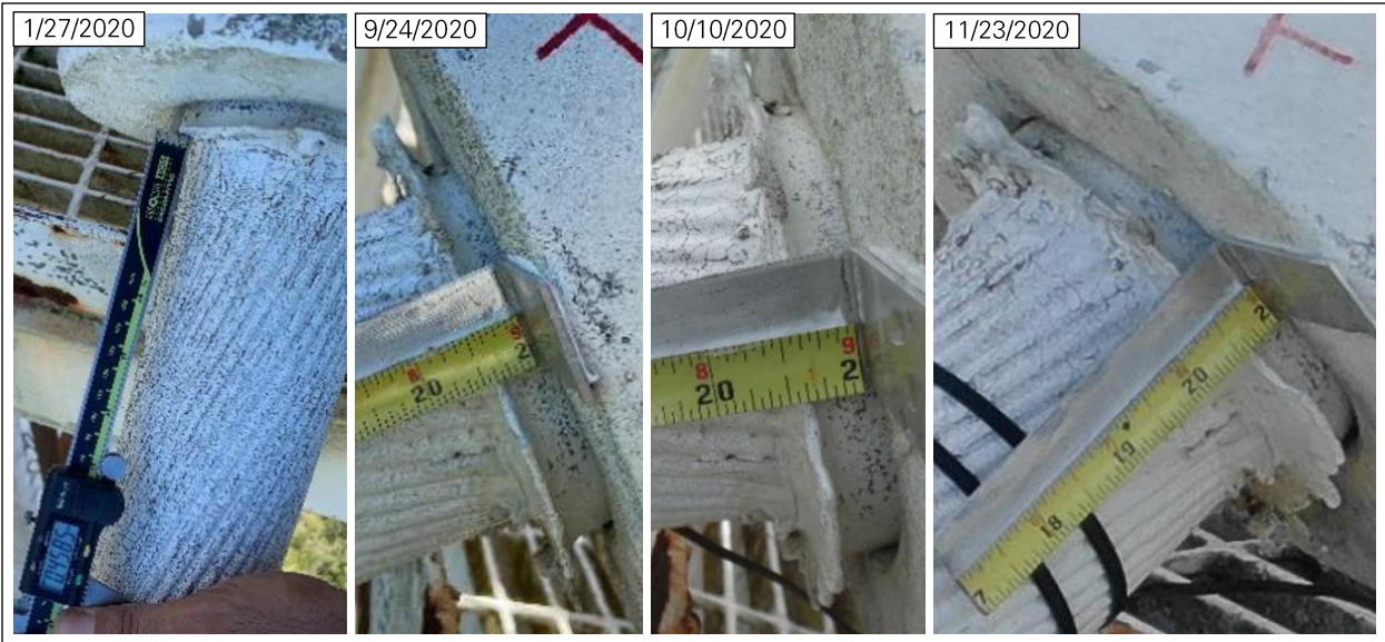
Figure 37: Cable slip at socket B12W_T (left and right photos: NAIC Arecibo Observatory, a facility of the NSF; center photos: WJE 14 ).
