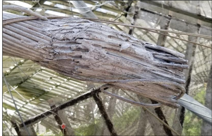
Figure 3: Cable end pulled out of socket M4N_T.
