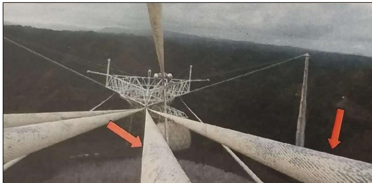
Figure 5: Paint deterioration on original mains at top of Tower 12 in 2011 ( photo: Ammann & Whitney 2 ).
