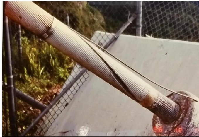
Figure 10: Wire break at ground end on B4-1 discovered on December 12, 1996 (photo: NAIC Arecibo Observatory, a facility of the NSF).
