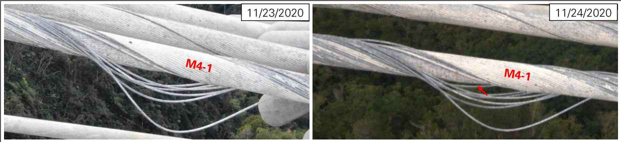
Figure 24: New wire break in M4-1 on November 20, 2020 (photos: NAIC Arecibo Observatory, a facility of the NSF).
