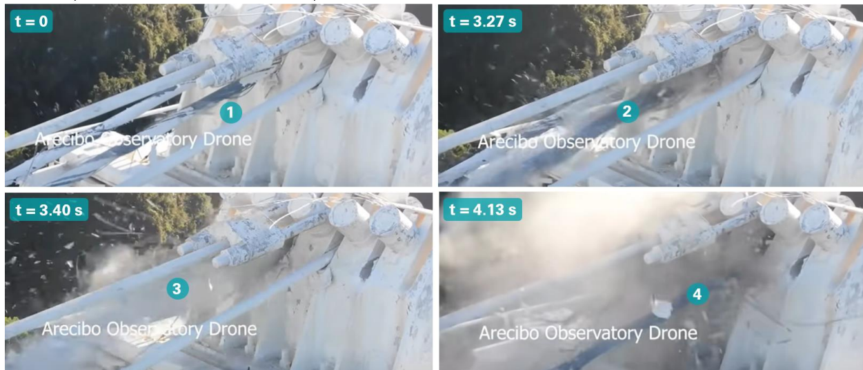
Figure 29: Progressive failure of original main cables at top of Tower 4. (still images of drone video by NAIC Arecibo Observatory, a facility of the NSF. Intermediate still images are provided in Appendix E.)
