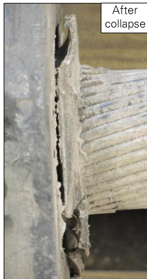
Figure 27: Cable slip at socket M4S_P.
