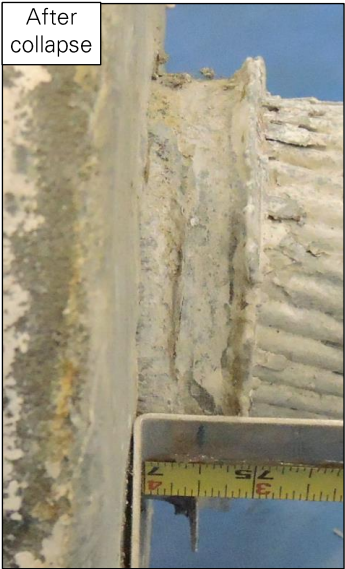
Figure 39: Cable slip at socket B4S_G.
