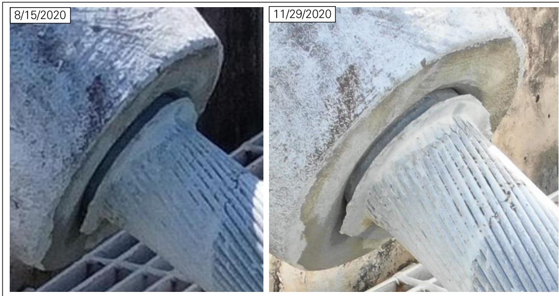
Figure 34: Cable slip at socket B8N_T (photos: NAIC Arecibo Observatory, a facility of the NSF).
