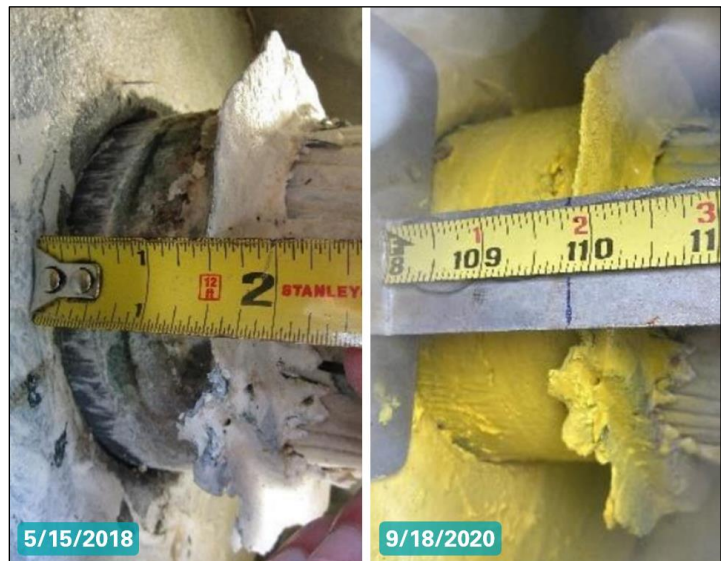
Figure 24: Cable slip increase measured at socket B12W_G (photos: NAIC Arecibo Observatory, a facility of the NSF).
