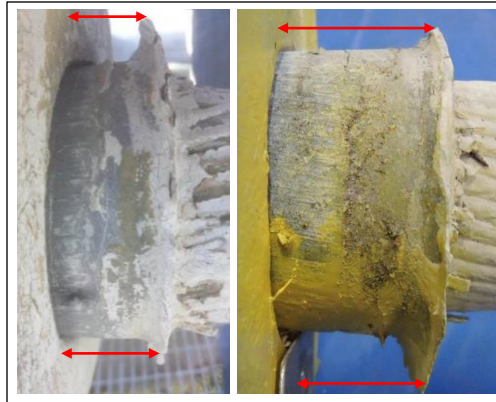
Figure 16: Cable slip at socket M4N_T (left) and B12W_G (right) (photos: NAIC Arecibo Observatory, a facility of the NSF).
