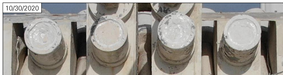
Figure 15: M4 sockets at Tower 4 on October 30, 2020. No significant change is visible since October 1, 2020. (Photo: NAIC Arecibo Observatory, a facility of the NSF.)
