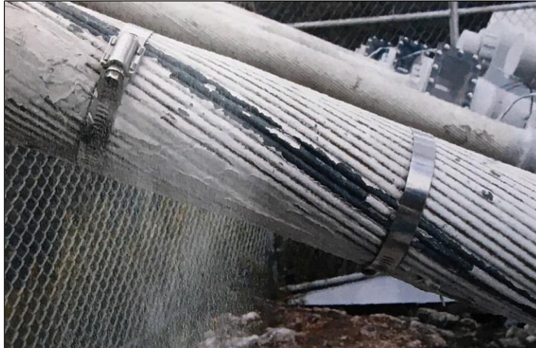
Figure 4: Original backstay B12-5 near anchor in 2003. Clamps and missing paint indicate a broken wire. Paint is also cracked between other wires ( photo: Ammann & Whitney 1 ).
