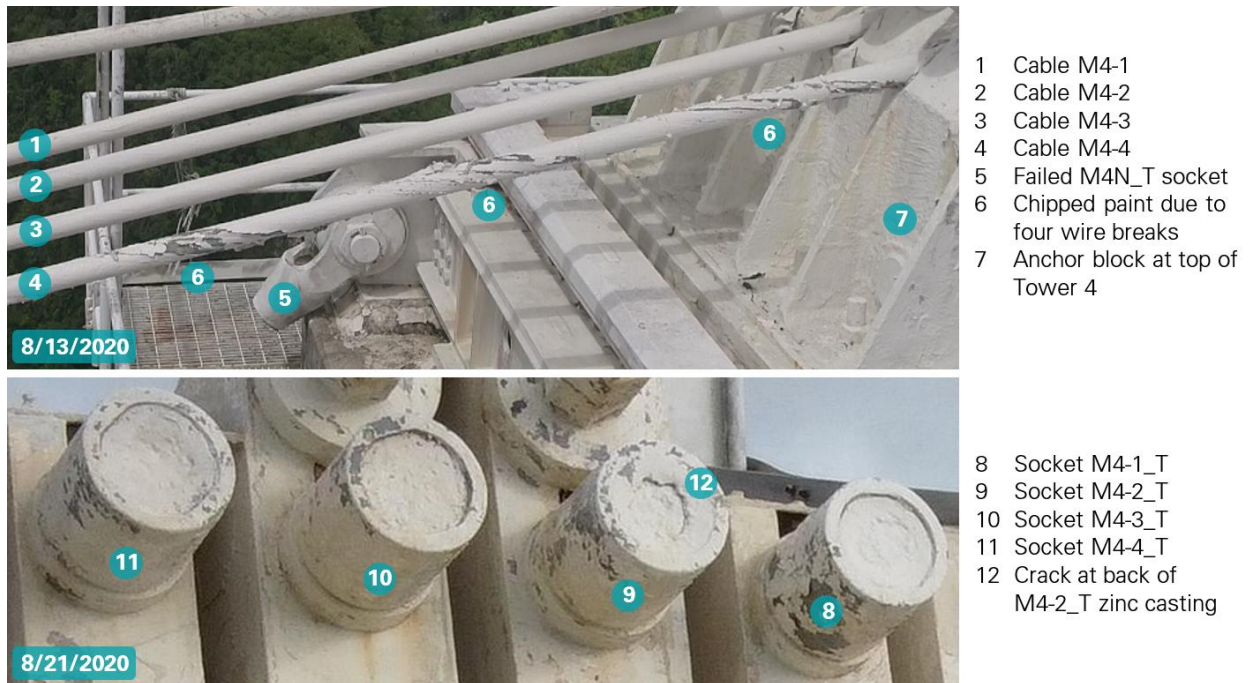
Figure 26: Damage on original M4 cables at top of Tower 4 after first cable failure (photos: NAIC Arecibo Observatory, a facility of the NSF).
