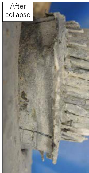
Figure 42: Cable slip at socket B12E_G.
