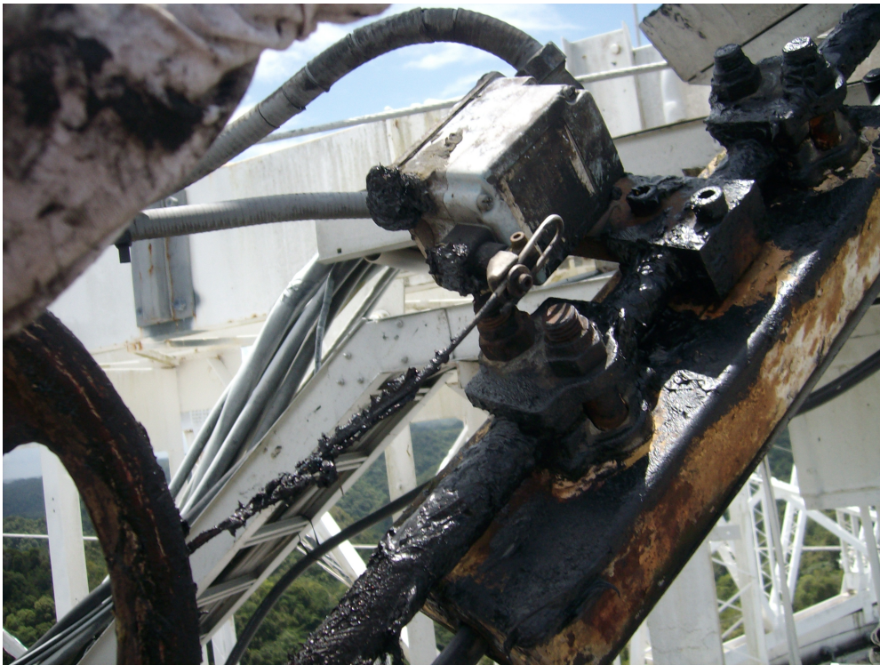
Photo 1 – Incorrectly located travel switch at upper terminal.
