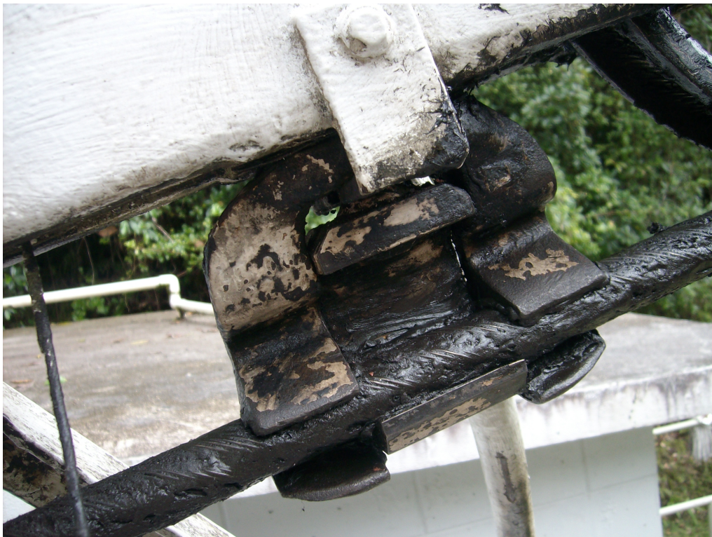
Photo 8 – Grip jaws of track rope brake clamp on to track rope but do not stop or hold
