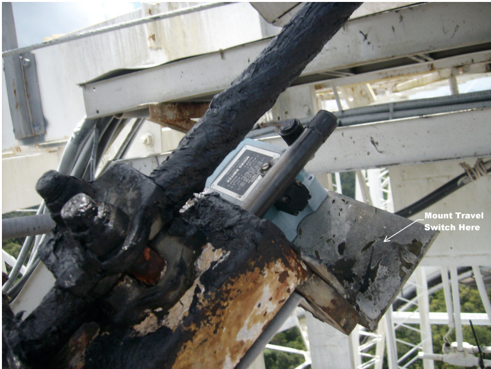
Photo 2 – Location to mount incorrectly located travel switch.
